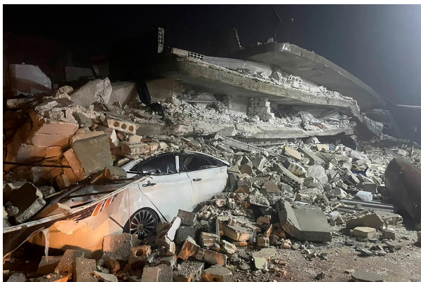
The consequences of the earthquake in Idlib.
